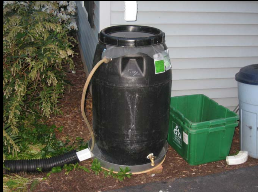
Barrel with overflow hose
